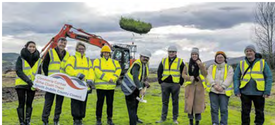
Pictured Mayor of SDCC Cllr. Baby Pereppadan with Teresa Walsh (SDCC Director of Service, Suzanne Furlong, Sean Redmond, Keith (Tim Austen Design), Shea McElhatton (ACS Civils Ltd) & SDCC staff at the sod turning for the Phase 2 works in Kiltipper Park. Pic credit: Ben Ryan
